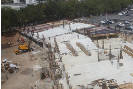
Construction of 4-level 500-vehicle parking garage at Federico Degetau Federal Building Photo: www.gsa.gov
